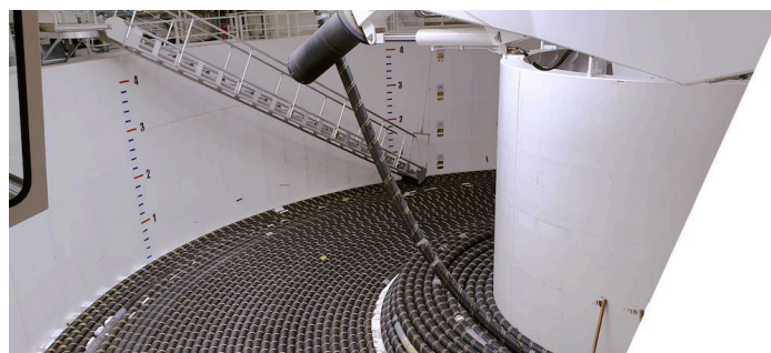
Typical power cables carried in a cable laying vessel (CLV).
